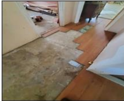
Damage d Floor
