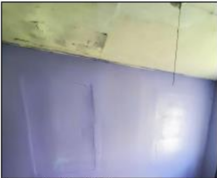
Damaged wall and Ceiling
