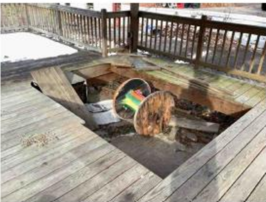
Covered Deck W/O Safety Railing
