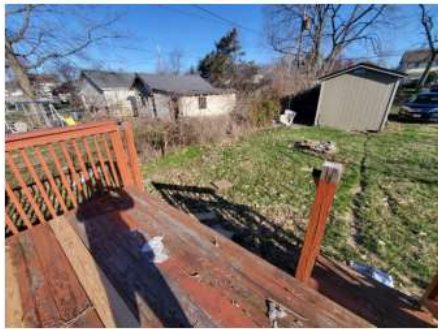
Missing Guard Railing around Deck
