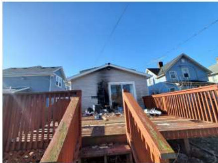
Peeling Paint - Deck
