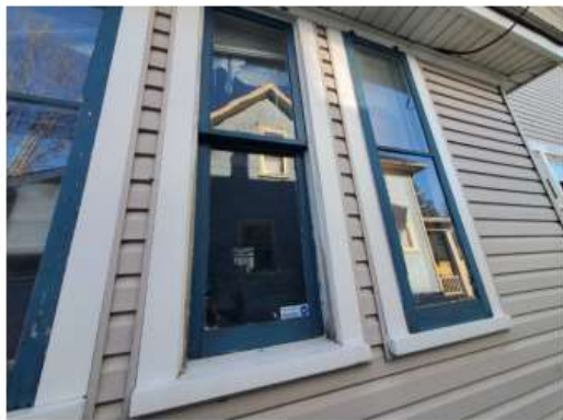
Peeling Paint - Exterior Windows
