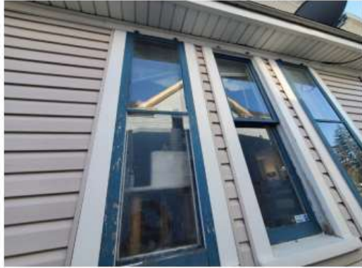
Peeling Paint - Exterior Windows
