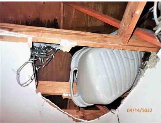
Damaged Ceiling In Garage With Items Hanging From The Attic
