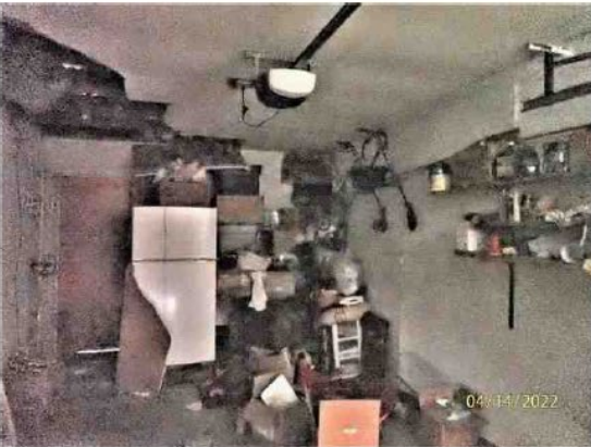
Garage With Damaged Ceiling On The Left
