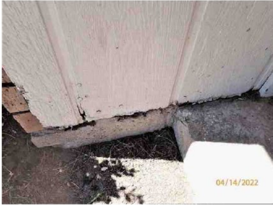
Deteriorated Exterior Siding
