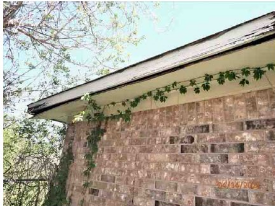
Soffits & Fascia Need Replacing & Paint
