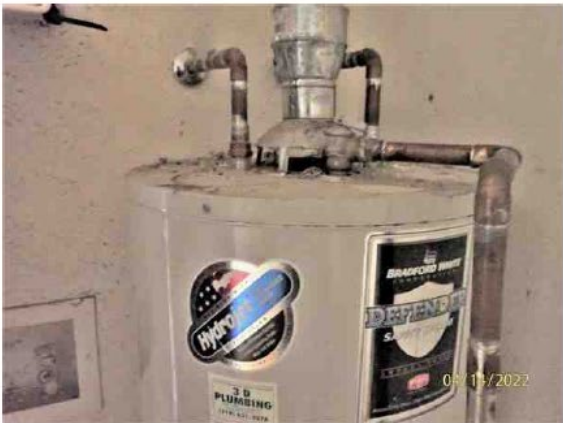
Gas Water Heater
