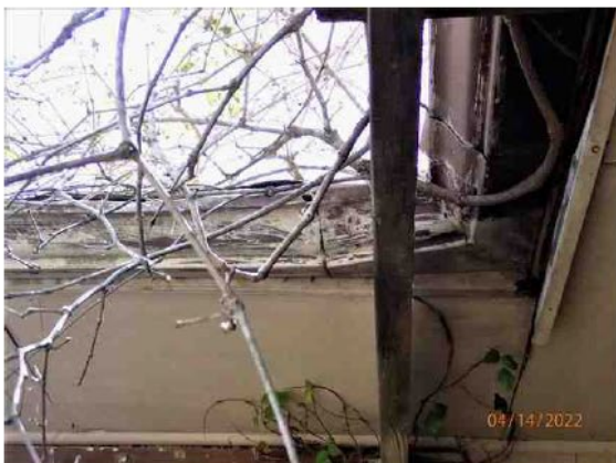
Damages To Soffits, Fascia & Gutters
