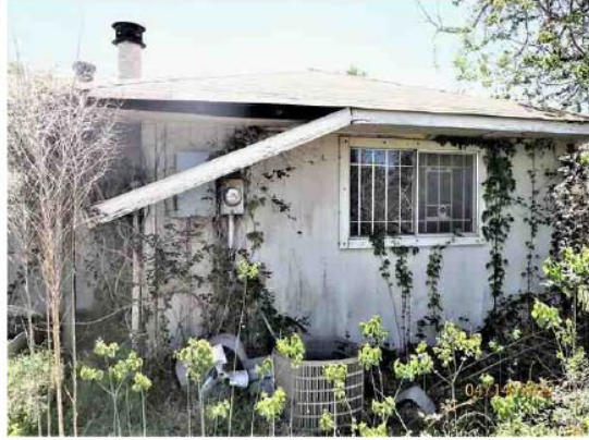
Damages To Exterior Siding, Soffits, Fascia
