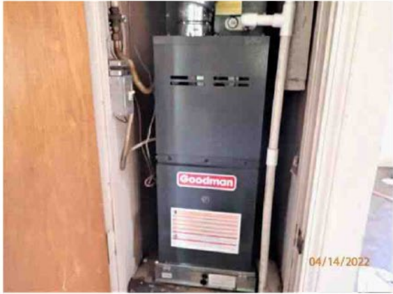
Gas Heating Furnace
