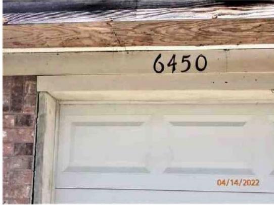
Wood Soffits & Fascia Need Paint; Possible Foundation Settlement As Evidenced By Opening Between Garage Door & Brick Wall
