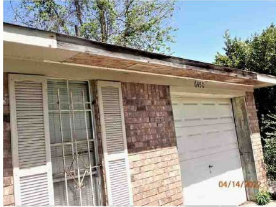
Wood Soffits, Fascia, Shutters & Iron Window Bars Need Paint.
