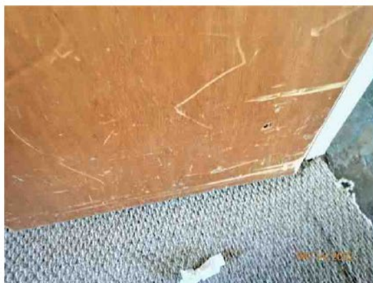
Damaged Interior Hollow Core Door & Floor Covering
