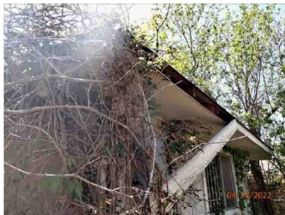
Damages To Soffits, Fascia & Gutters
