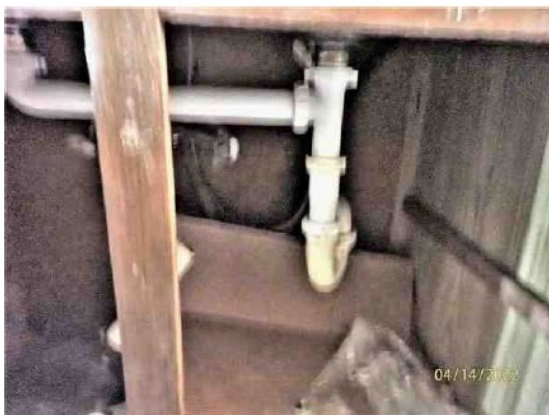
Interior Of Kitchen Sink Cabinet & Plumbing
