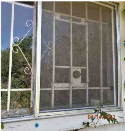
Safety Pop-Out Security Window Irons On Bedroom Windows Need Paint
