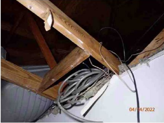
View Of Attic & Wiring Through Damaged Ceiling In Garage
