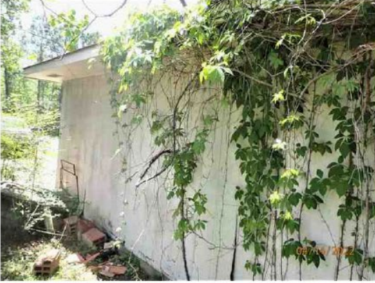
Tree & Foliage Growth Causing Damages To Exterior Siding, Soffits, Fascia & Roof
