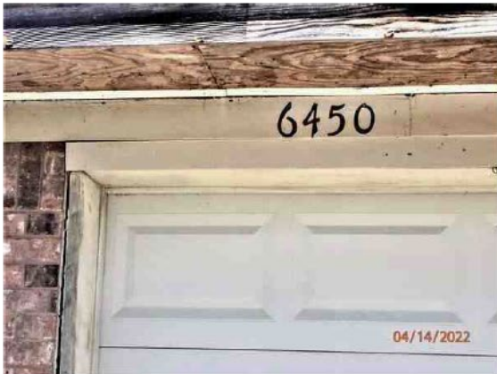
Gap Between Garage Door Frame & Brick Wall Indicates Possible Foundation Settlement
