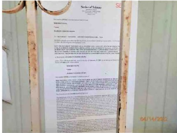
Notice Of Seizure & Iron Door Needing Paint
