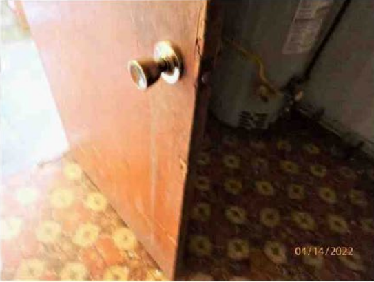
Damaged Interior Hollow Core Door
