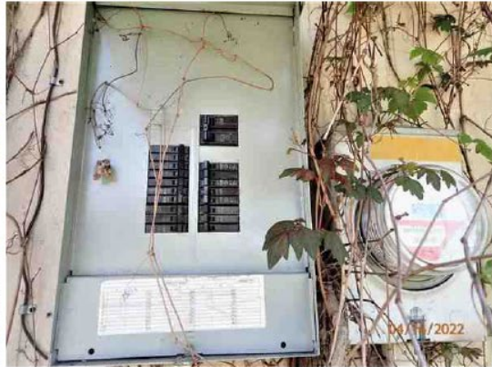
Electric Service Panel
