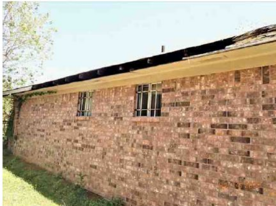
Soffits & Fascia Need Replacing & Paint: Window Irons Need Paint
