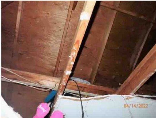
Damaged Ceiling In Garage
