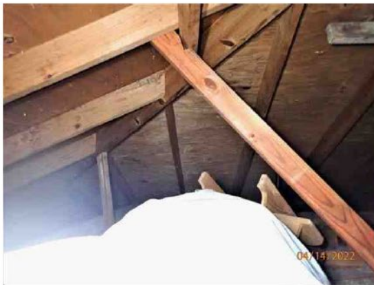
View Of Attic Through Damaged Ceiling In Garage
