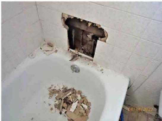
Plumbing Damages To Bathtub
