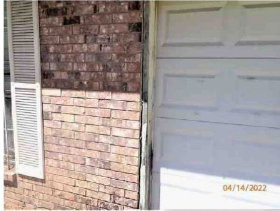
Deteriorated Garage Door Frame
