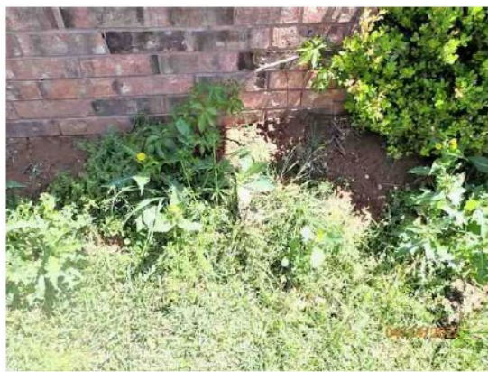
Dirt Mounds Around Foundation May Be Hiding Soil Subsidence Or Foundation Settlement
